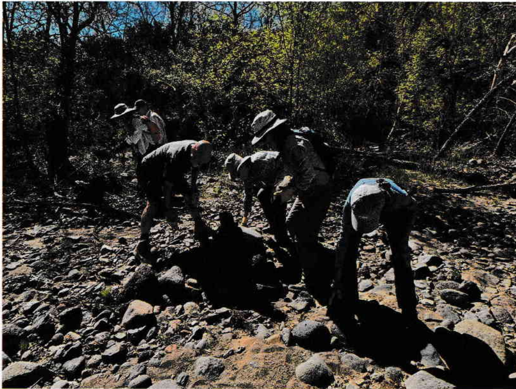
Friends of the Tonto National Forest repair damage on the Sheep Creek Trail
